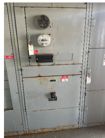
Existing Electric Service
